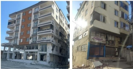
Figure 4. Overhang buildings in Hatay after on February 6, 2023, Kahramanmaraş earthquake
