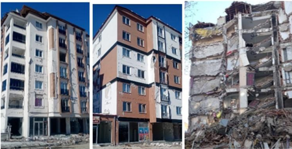
Figure 3. Overhang buildings in Malatya after on February 6, 2023, Kahramanmaraş earthquake
